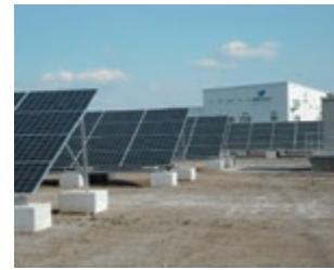
Photovoltaic power plant of RIKEN TECHNOS CORPORATION (within the Gunma Factory site)
